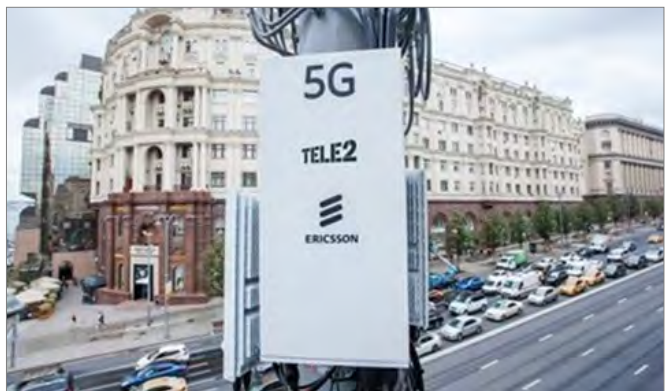
Figure 7: Ericsson 5G micro base station in an urban environment (photo: Ericsson)
